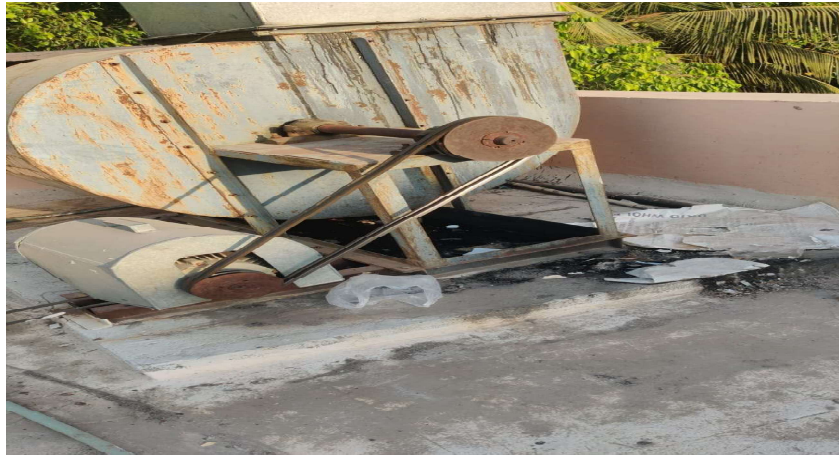
Figure 7. Image of belt-driven kitchen exhaust
