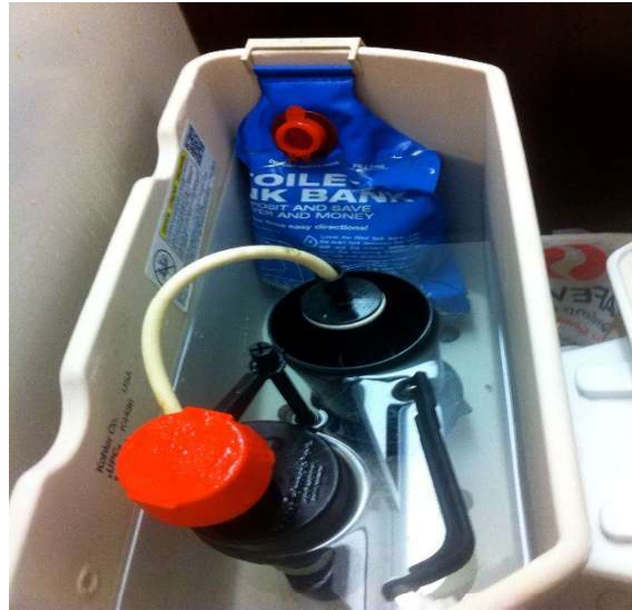
Figure 12. Flush toilet tank bank
